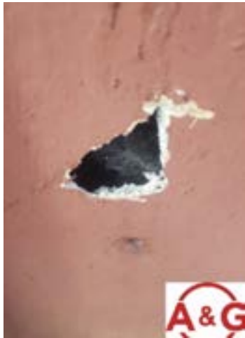
Fibras sueltas (borra de amianto)
